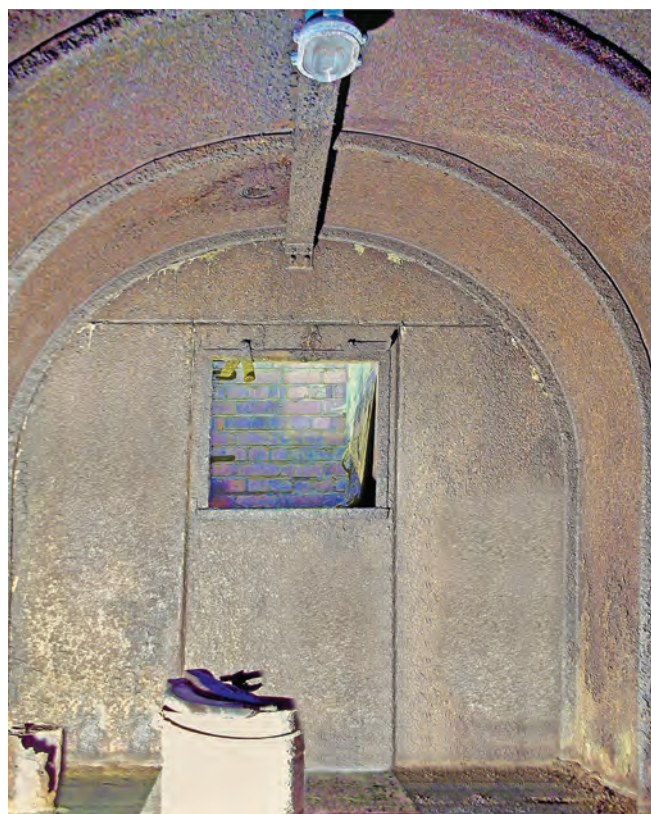
Looking towards the emergency exit with step-irons (seen on the left) up to a hatch in the garden. A Wigan bulkhead light is seen fixed to the ceiling. The air vent can just be made out in the ceiling.
